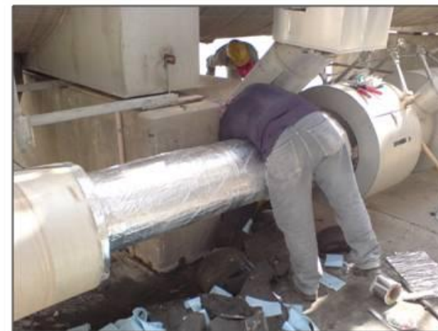
Broken pieces of traditional insulation. Minimal access.
